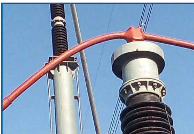
Substation installed with IEP Products
