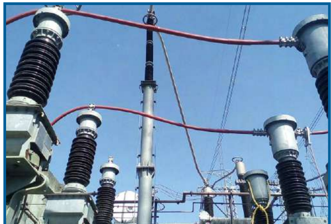
Substation installed with IEP Products
