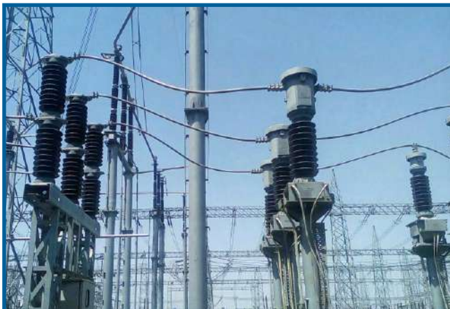
Substation without IEP Products
