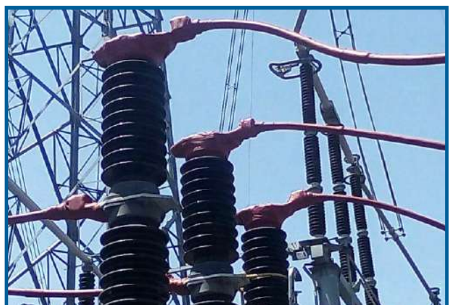
Substation installed with IEP Products
